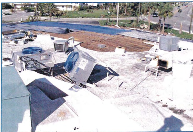
Figure 1 – Hurricane Charley, 2004: Edge flashing damage initiates roof blow-off. Photo courtesy of RICOWI.
