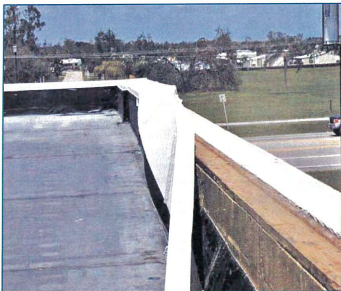
Figure 4 – Hurricane Charley, 2004: Coping blow-off. Photo courtesy of RICOWI.
